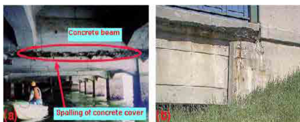
Fig 6. Corrosion of reinforced concrete. (a) Seawater structure; (b) bridge structure on highway 401 in Ontario, Canada (adapted from Refs [22] and [23], respectively).
