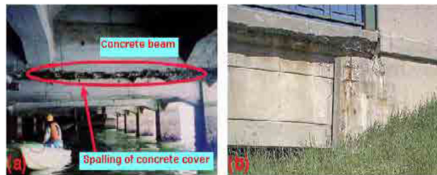
Fig 6. Corrosion of reinforced concrete. (a) Seawater structure; (b) bridge structure on highway 401 in Ontario, Canada (adapted from Refs [22] and [23], respectively).
